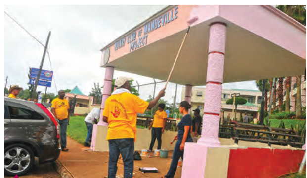
#VMProud Volunteers giving the Mandeville Hospital Bus Bay a much needed transformation.
